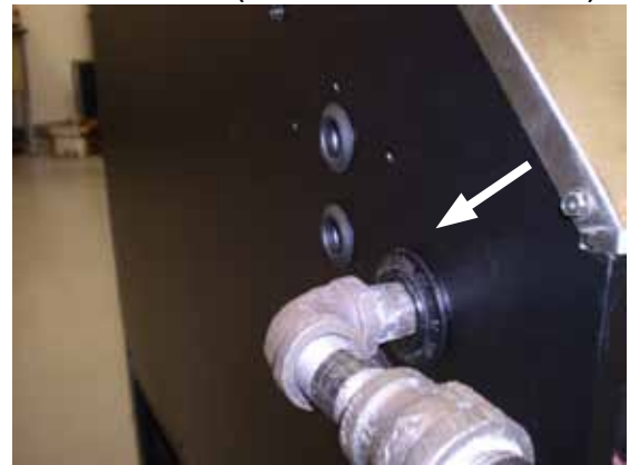
FIGURE 28 - FURNACE GAS PIPE CONNECTIONS (NOTE RUBBER GROMMET)
