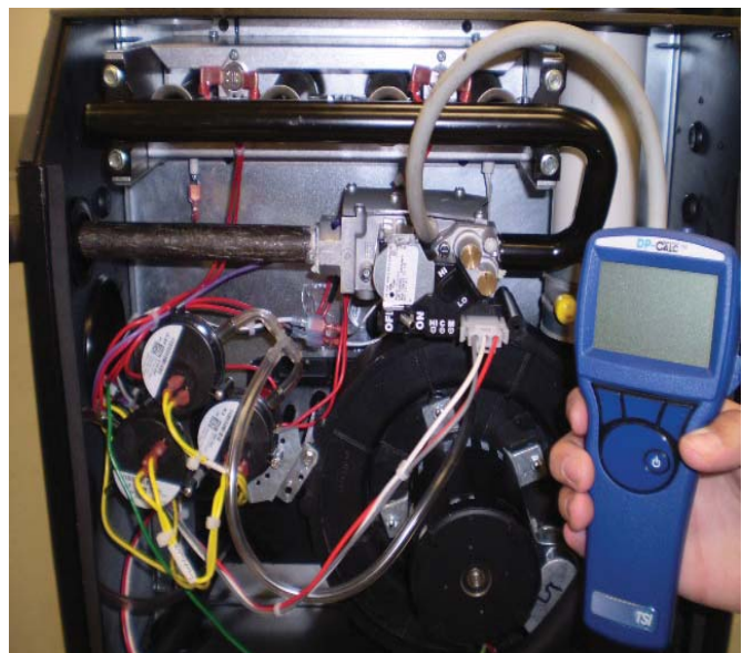
FIGURE 30 - MANOMETER MEASURING GAS MANIFOLD PRESSURE
